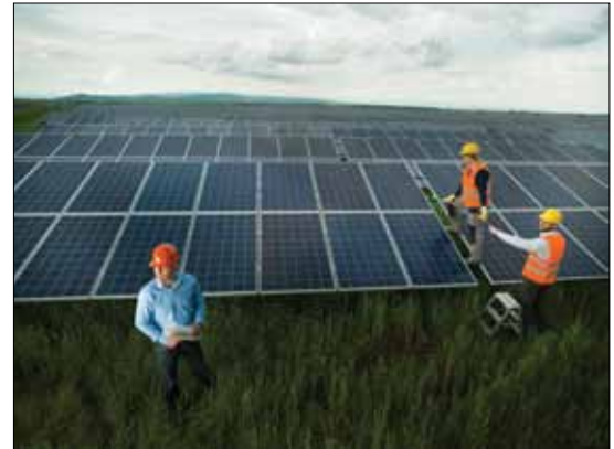
Utility scale solar project.
