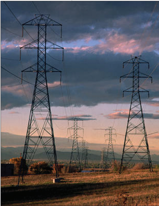
Transmission lines transmitting power. Photo by FERC.
