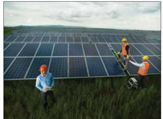
Utility scale solar project.
